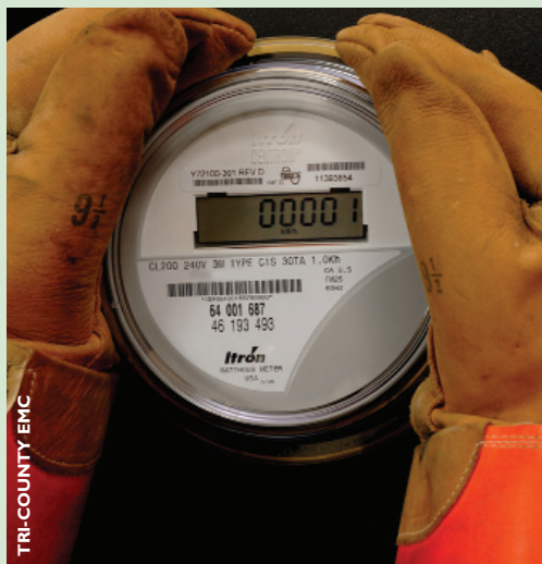
Smart meters enable consumers to participate in cost-cutting programs by shifting some energy use to off-peak periods.
